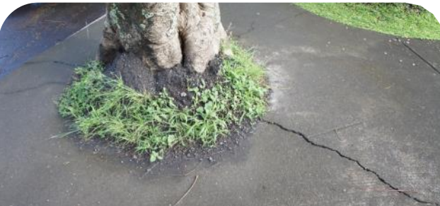
Fig. E6.1 Pavement damage due to large root spread and insufficient space between the pavement and tree trunk
