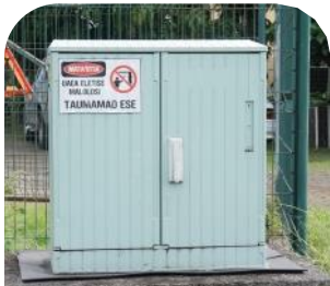
Fig. C6.1 Adequate enclosure and warning sign
