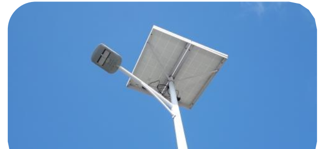
Fig. E5.3 Solar-powered street lighting
